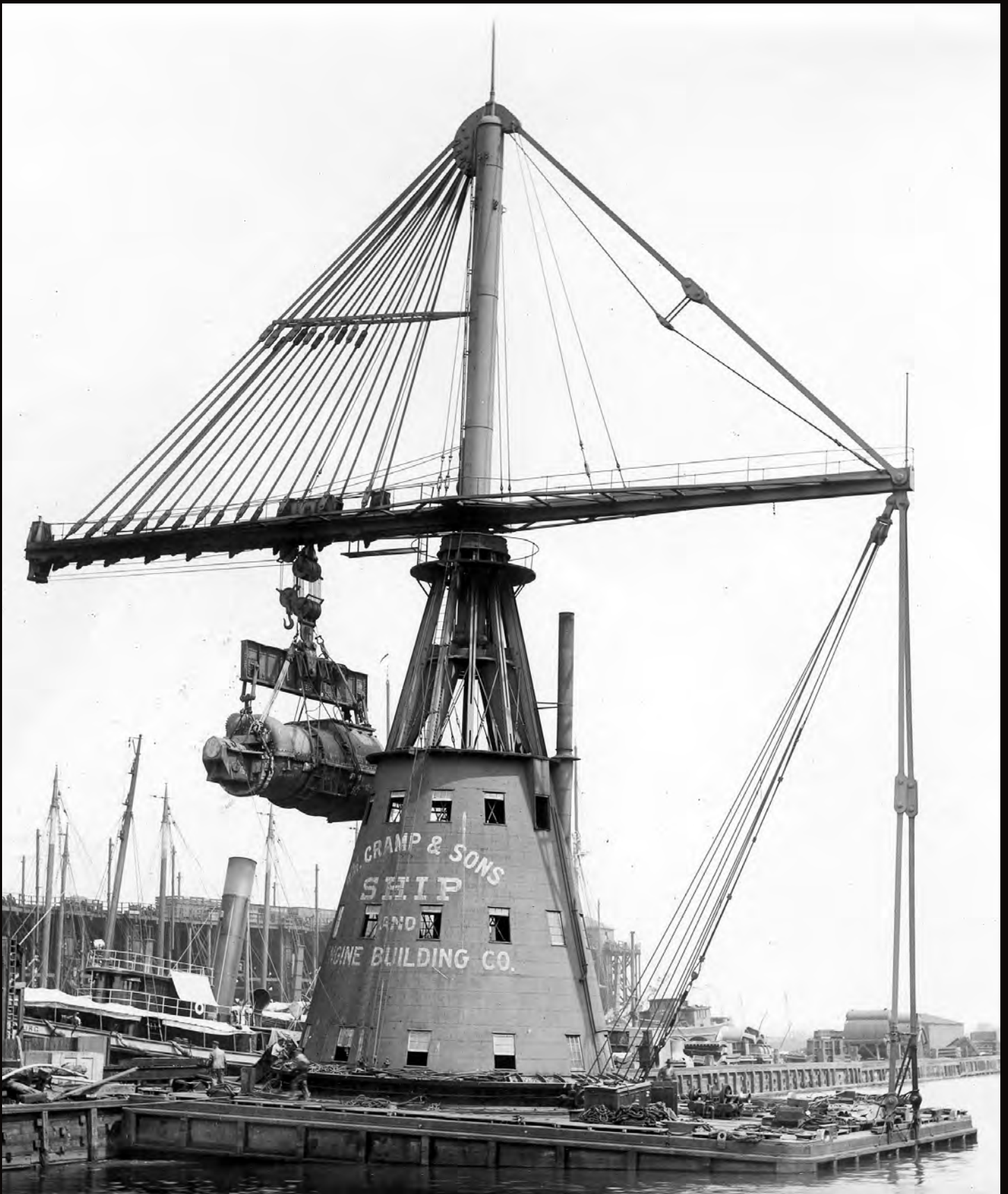
Huge floating crane carrying one of three Parsons steam turbine engines for installation on the Great Northern . Each of these engines weighed 197,000 pounds or 98.5 tons and was manufactured by Cramp & Sons under license from inventor Charles H. Parsons. CRMM 411-9386
